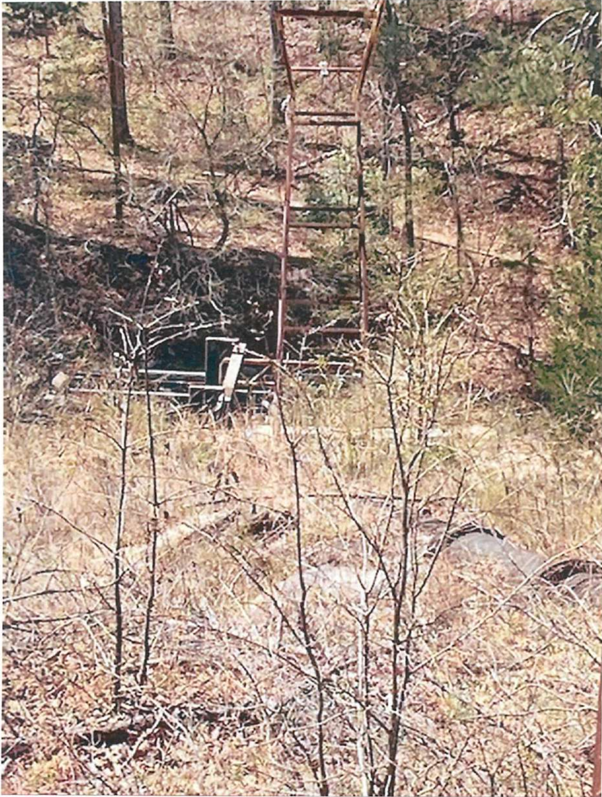
This is a view from the top of the hill where the check valve building is located down to the mezzanine where the pumps & motors are located. The 24" water line is partially underground.
